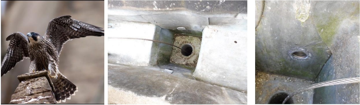
Views of lead hopper gutters with internal lead burning to the new overflow pipes – the sumps have previously been blocked by carrion dropped by the peregrine falcons.
