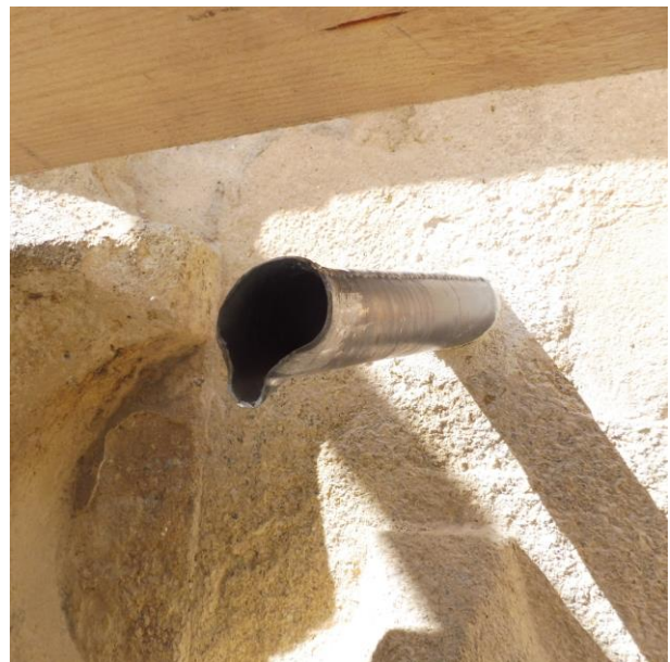
Close up of lead overflow pipe
