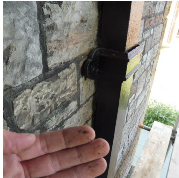
Back of this downpipe was rusted through
